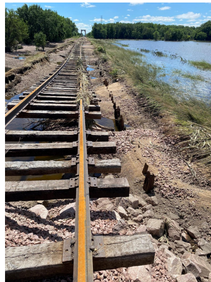
Washout showing missing ties and high potential of ties being lost during washout filling operations
