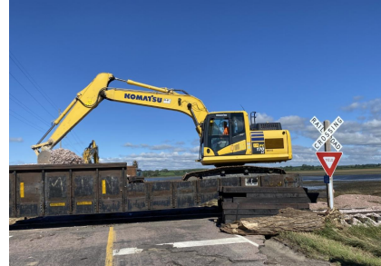
Modified gondola railcar - Excavator end of car is pushed to washout, where it placed rock from the car into the washout.
